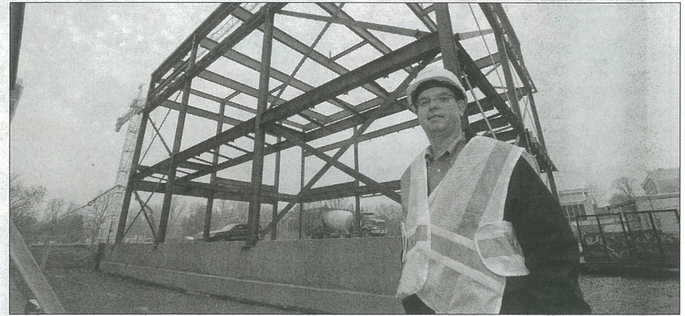
Work on the Burlington Performing Arts Centre is progressing on time and within budget according to project manager Craig Stevens (pictured). Steel structures are in place and walls are going up as construction continues through the fall and winter months
